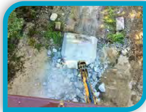
View from above, as District staff use a hoe ram to remove a concrete bridge pier and deck lying in the Carmel River.
