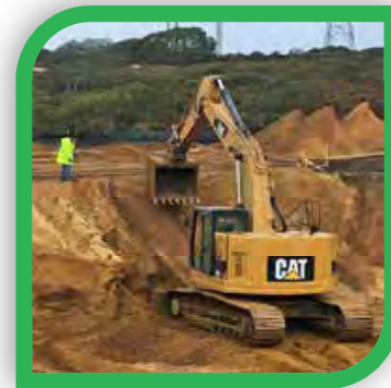
Construction of expanded percolation pond to accommodate waters from four existing and two future ASR wells.
